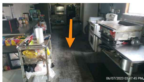
Dip in Flooring
