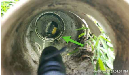
Right Side Clean-Out
