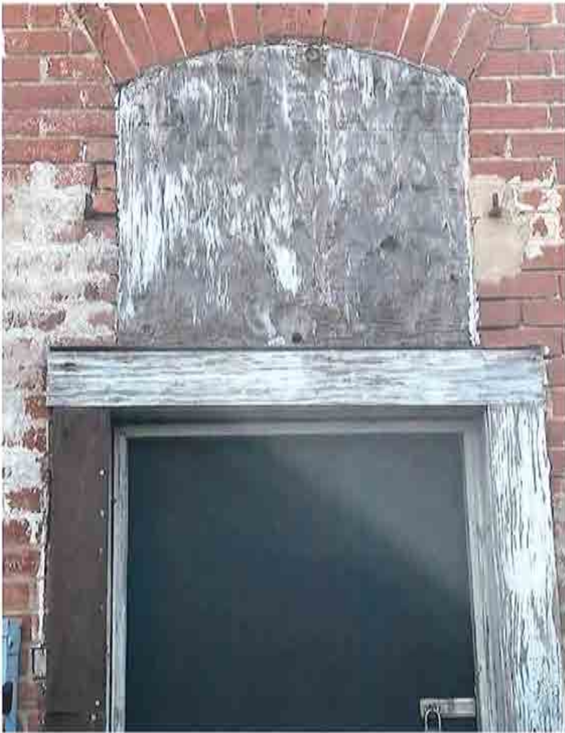
Back Exit Door 225 Fowlkes Masonry infill above door and a new door
